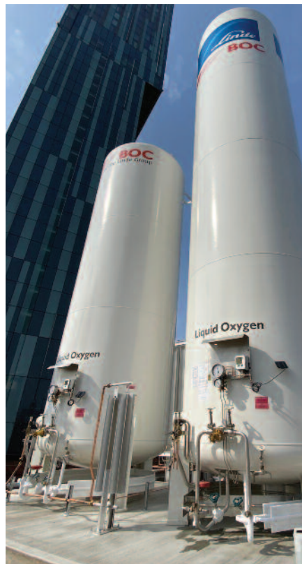
It was agreed that the site needed at least one vacuum insulated evaporator (VIE) unit.
